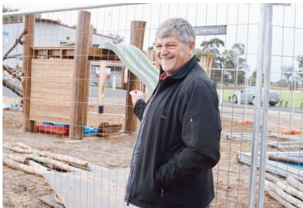
PLAYGROUND ON ITS WAY: McCorquindale Park committee member Leigh Miller examines the ongoing installation of the new nature playground at the sporting hub.
