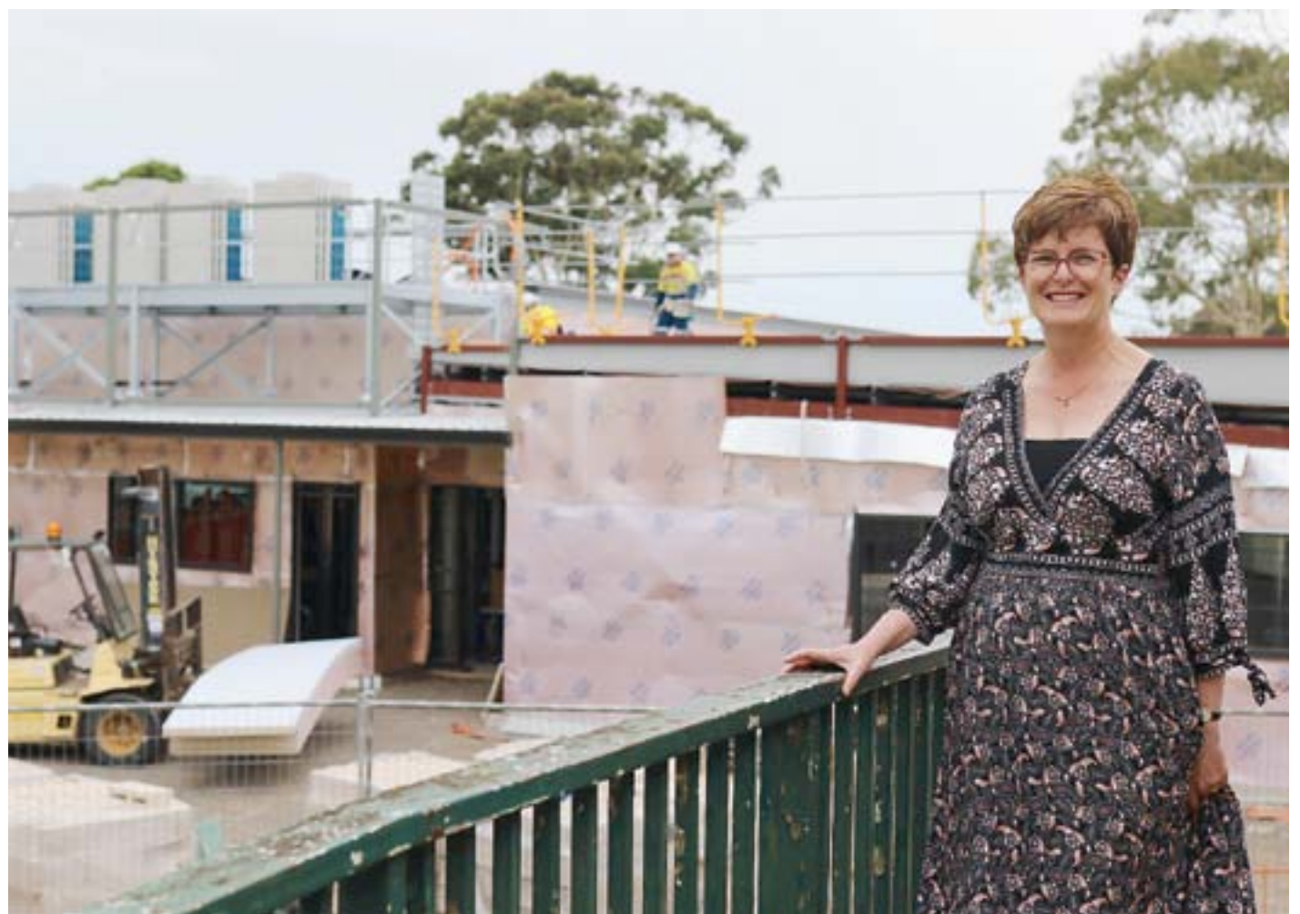
PROGRESSING WELL: Grant High School principal Fleur Roachock stands in front of the site's $7m development which is on track for its estimated end-of-year handover. Picture: MOLLY TAYLOR
