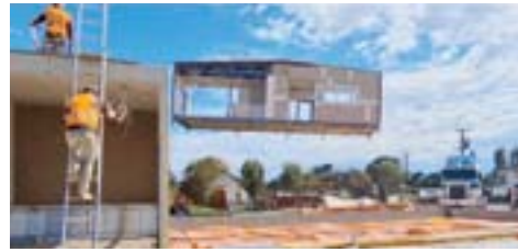
PRESCHOOL FROM THE SKY: One of six pre-fabricated modules which make up the new Moorak Preschool is craned into place this week.
