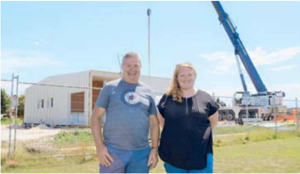
CRANED INTO PLACE: Moorak Primary School Principal Peter Mitchinson and Preschool Teacher Lauren Baudinette were on site to see the new Moorak Preschool buildings put in place this week.
