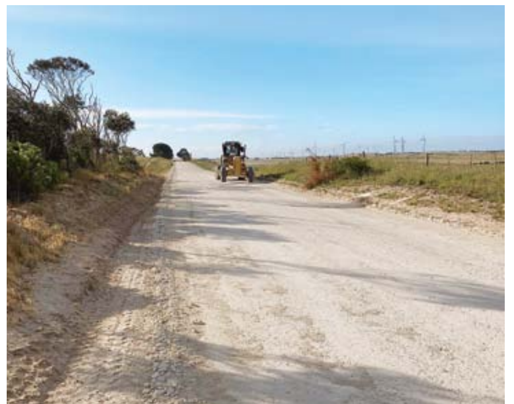
ROADWORKS UNDERWAY: Grader on Pinchgut Road in the Millicent area - one of several unsealed roads on Wattle Range Council's resheeting works program for the year. Picture: WATTLE RANGE COUNCIL
