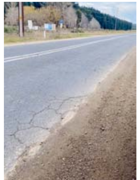
WORK NEEDED: Damage along Mile Hill Road.
