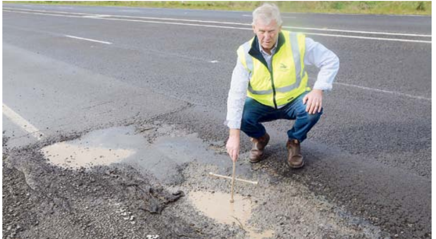
POTHOLE DANGER: Wattle Range mayor Des Noll examines one of the many potholes that have opened up on the Princes Highway.
