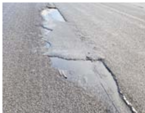
HIGHWAY OF HOLES: Geotextile road stabilisations that were applied to the Princes Highway in recent years have failed and sections of road are lifting as a result.
