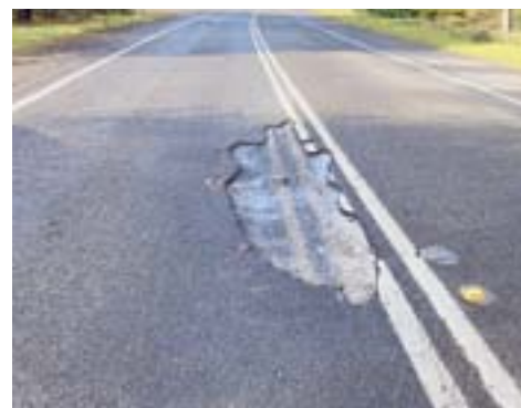
DANGER ZONE: Dozens of motorists have reported sustaining damage to vehicles due to hitting potholes along the Princes Highway.
